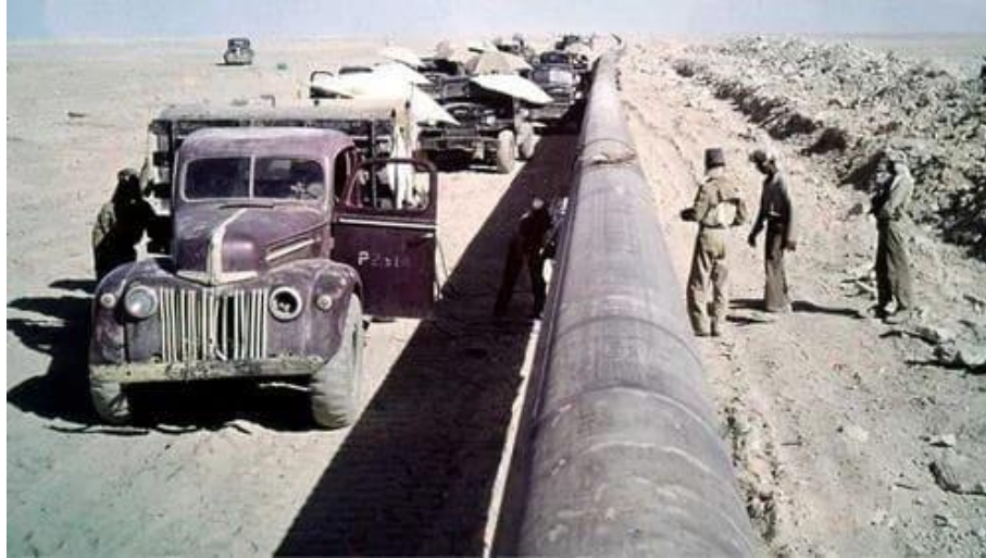
Fig. 10 200,000 steel tubes, each 9 meters long were used to construct the TAPLINE. Source: from Aramco (2021).
